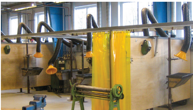
Wing arms \varnothing 160\text{mm} 3m installed at technical school. Including automatic control devices for automatic start/stop of fan and motor damper.
